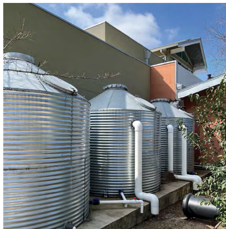
Eagle Veterinary Hospital has 3,000-gallon water reclamation tanks that collect rainwater and air conditioning condensate that then goes through charcoal/UV filters before re-entering the hospital. Courtesy of Eagle Veterinary Hospital
